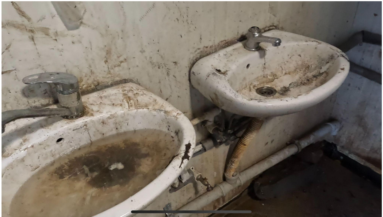
Sombor Camp, 17th January 2023, sinks in shared bathroom, 02:50
